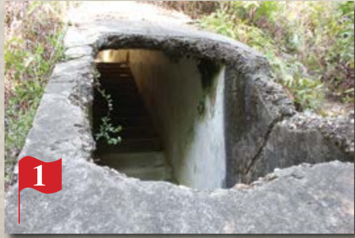
▲ 部分已損毀的隧道 A partially destroyed tunnel
